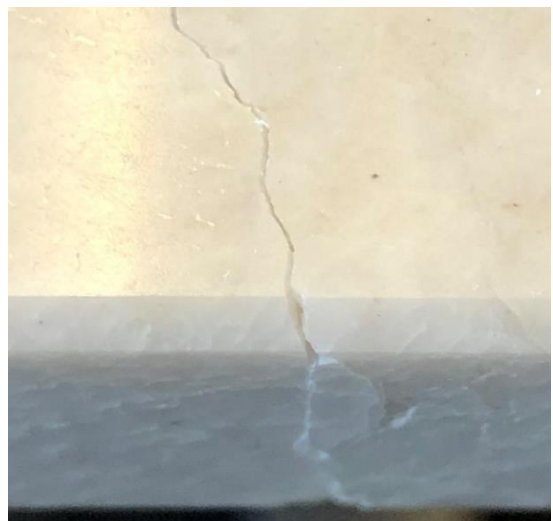
An example of a through-crack with a clearly visible gap between the fracture surfaces.
