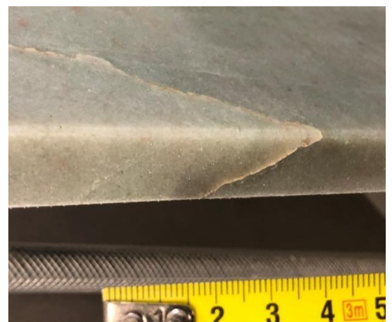
This image shows a vein, which may visually be mistaken for a crack.
